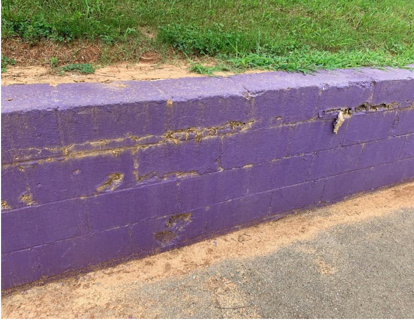
Deterioration of retaining wall along the Visitor side path to concessions.
