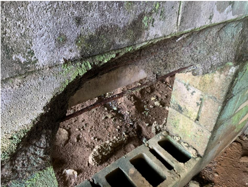
Loss of masonry and grout with exposed reinforcing in masonry lintel.
