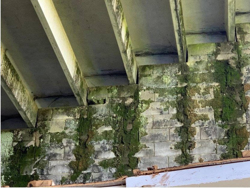
Water infiltration, moss growth, cracking and loss of section in interior masonry wall.
