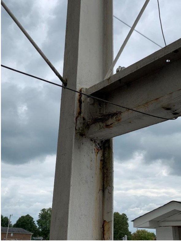
Rusting steel in the column support of the Home side press box.
