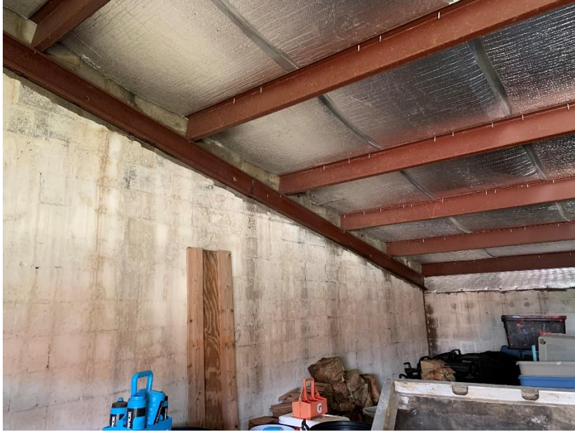
Interior masonry built-out space below Home side bleachers without water infiltration.
