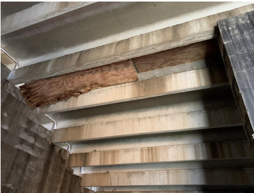
Previous repair to concrete plank and infill masonry wall providing intermediate support.
