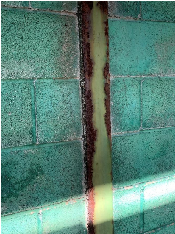
Corrosion of column flanges in contact with masonry walls.
