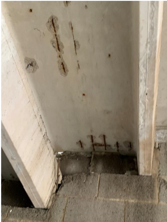
Underside of concrete plank with deterioration of the concrete and exposed steel reinforcing.
