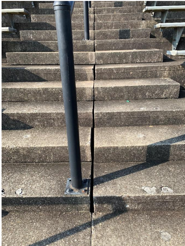
Absence of joint sealant between concrete planks.
