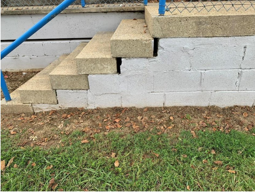
Egress steps requiring repair to realign the riser.
