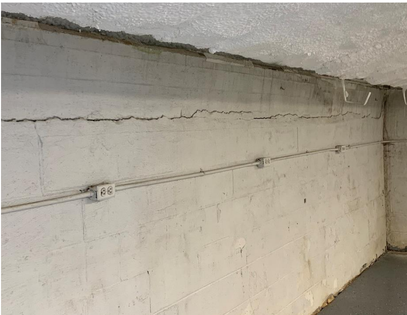
Cracking along the length of the top of the skirt wall along the front of the Home side bleachers.
