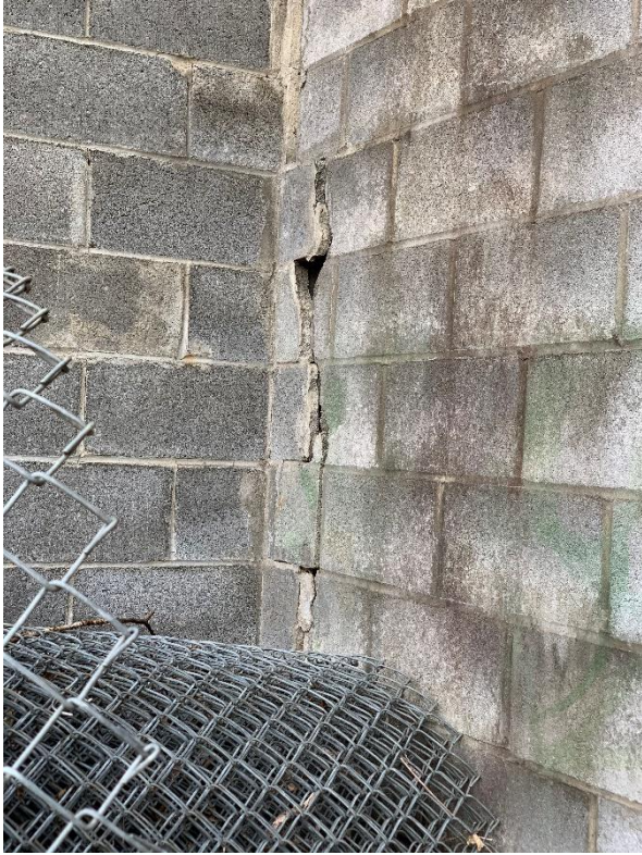
Crack in Visitor side rear wall requiring repair.
