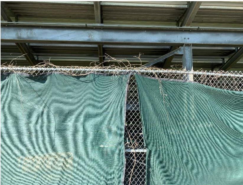
Evidence of invasive vegetation previously growing near the bleachers.
