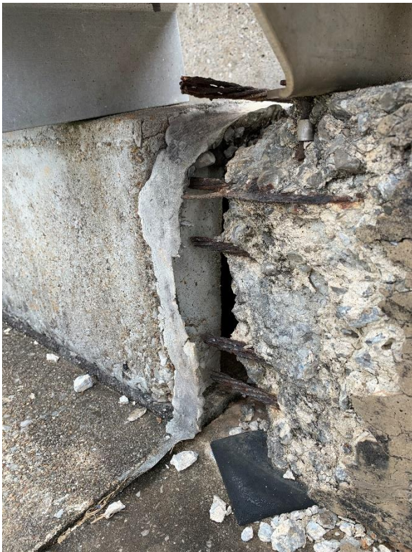
Example of deterioration in concrete plank with exposed reinforcing.
