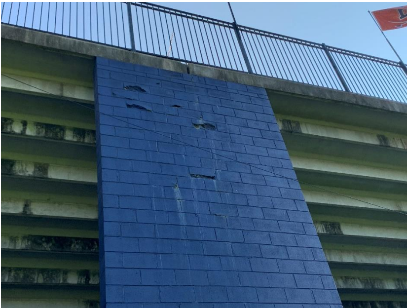
Spalling masonry along rear wall.
