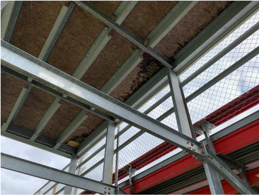
Water damage to the floor of the Visitor side press box.
