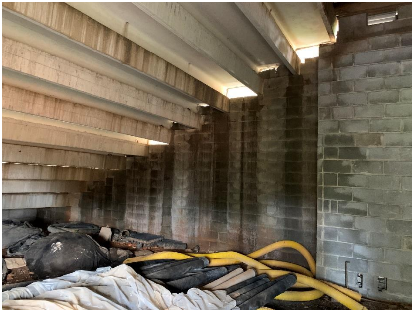
Example of missing block between stems of concrete planks to reduce water infiltration.
