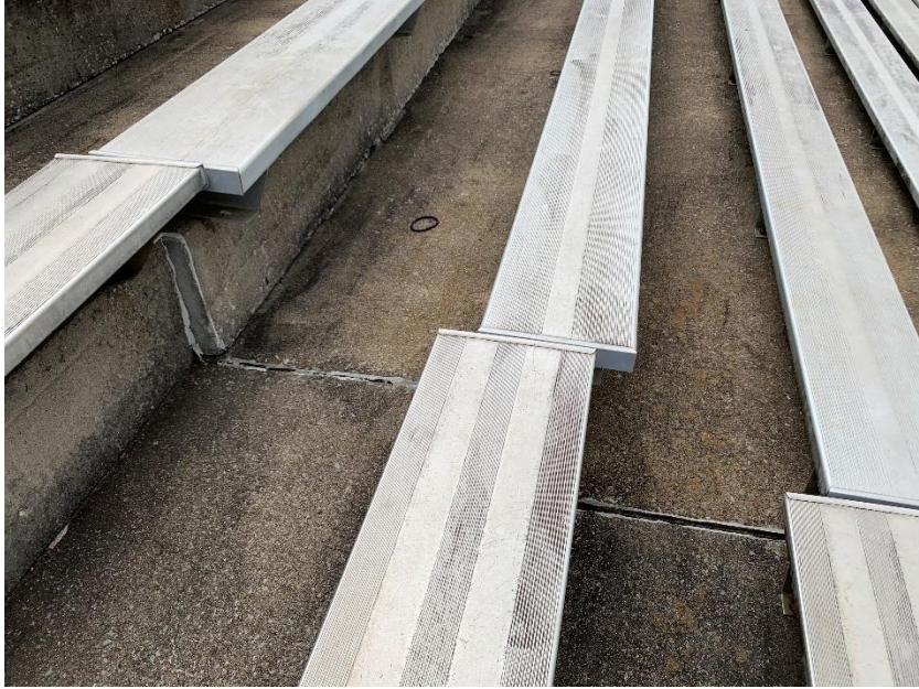
Far-right section of Home side bleachers with plank displacement.
