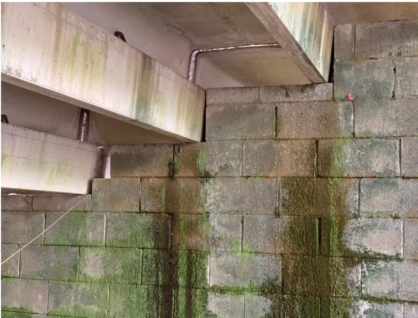
Interior Home side masonry walls with water infiltration and moss growth.
