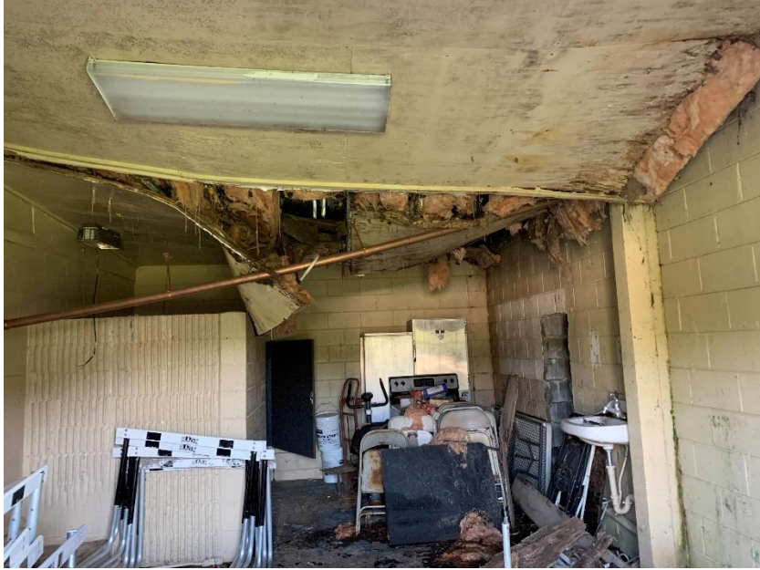
Water infiltration to built-out area beneath bleachers.
