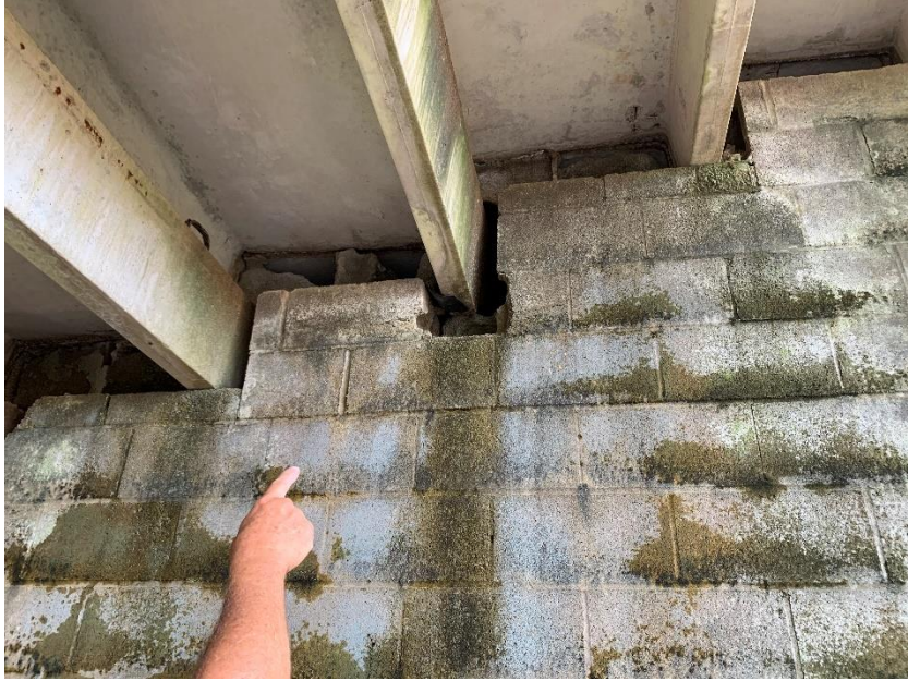
Example of concrete plank requiring masonry support on Visitor side bleachers.
