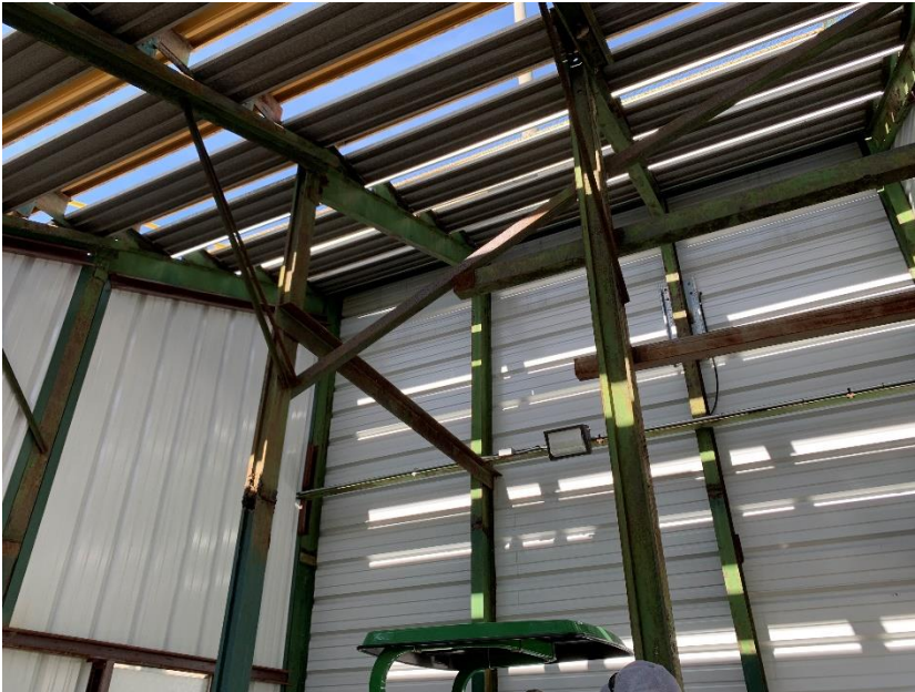
Example of interior framing with railroad rail columns and beams, and diagonal bracing.
