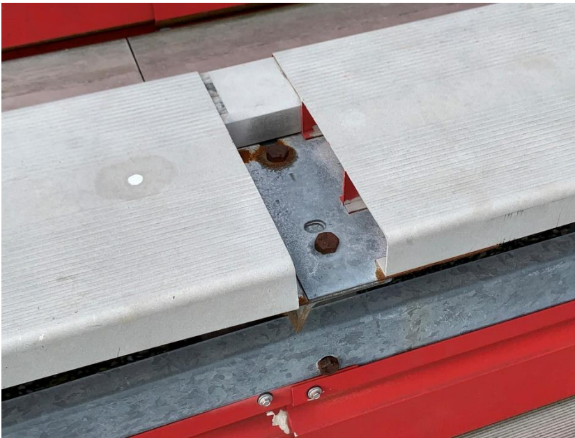
Example of rusted bolts needing replacement.
