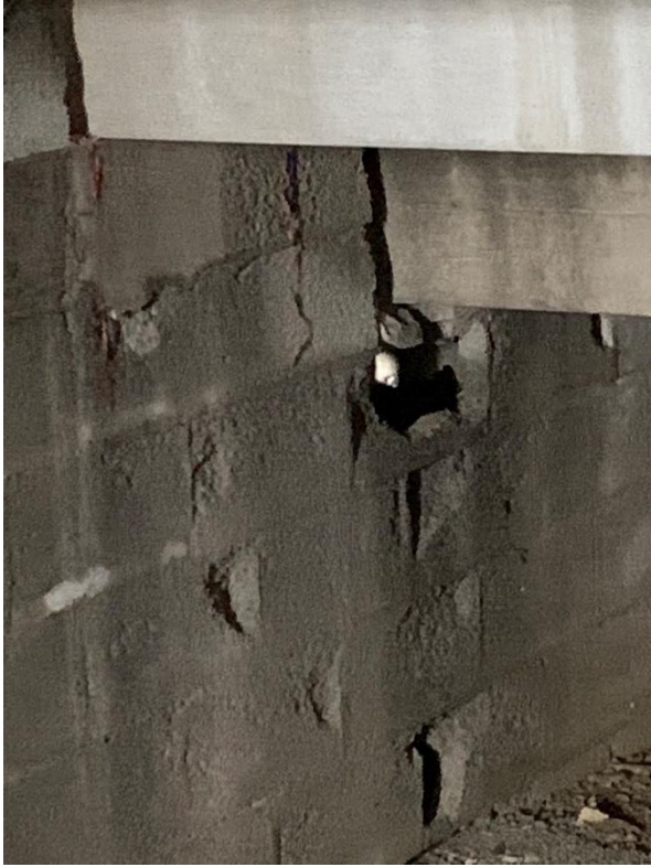
Extensive loss of section in Visitor side masonry wall.
