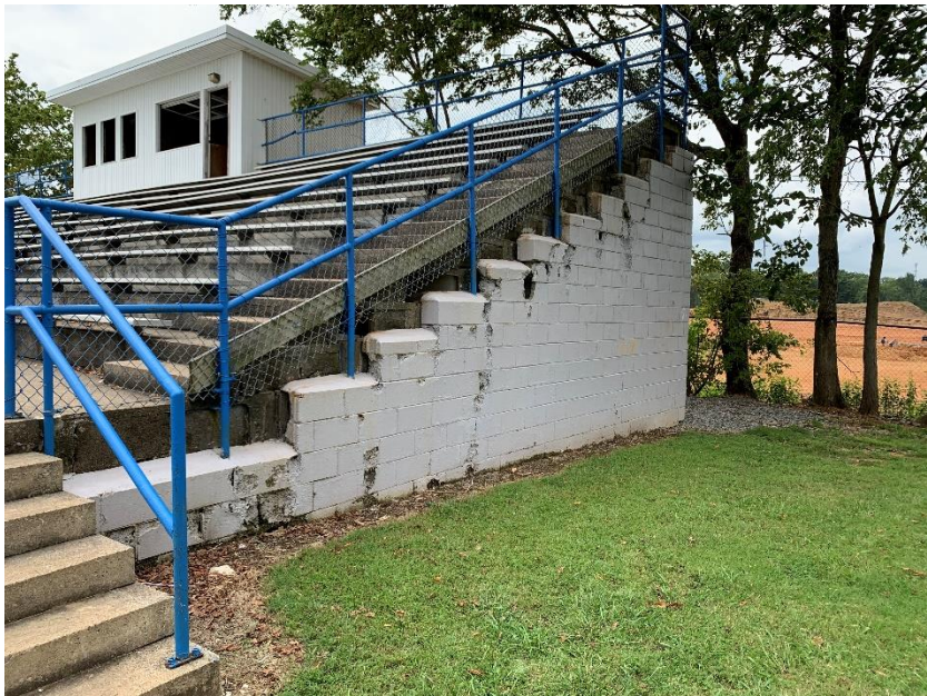
Visitors side bleachers with crumbling side wall supporting guardrail.
