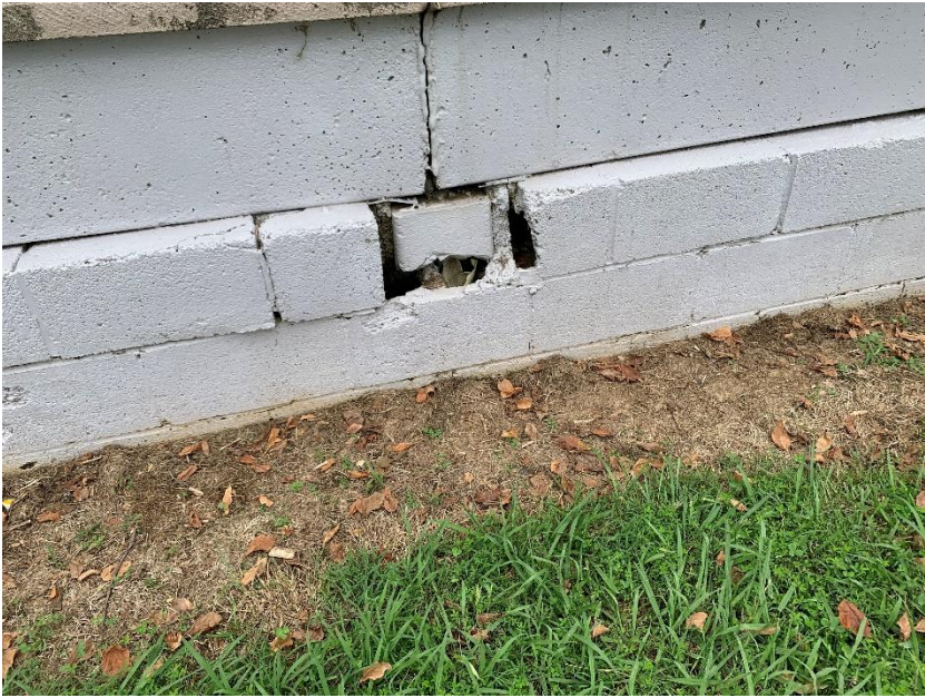
Location for repair front skirt wall at intersection of masonry support wall.
