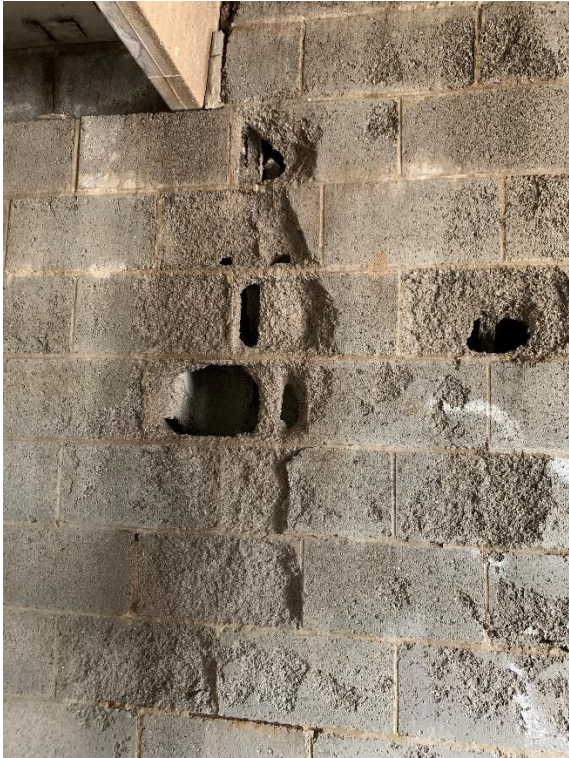
Home side masonry wall with extensive loss of section.
