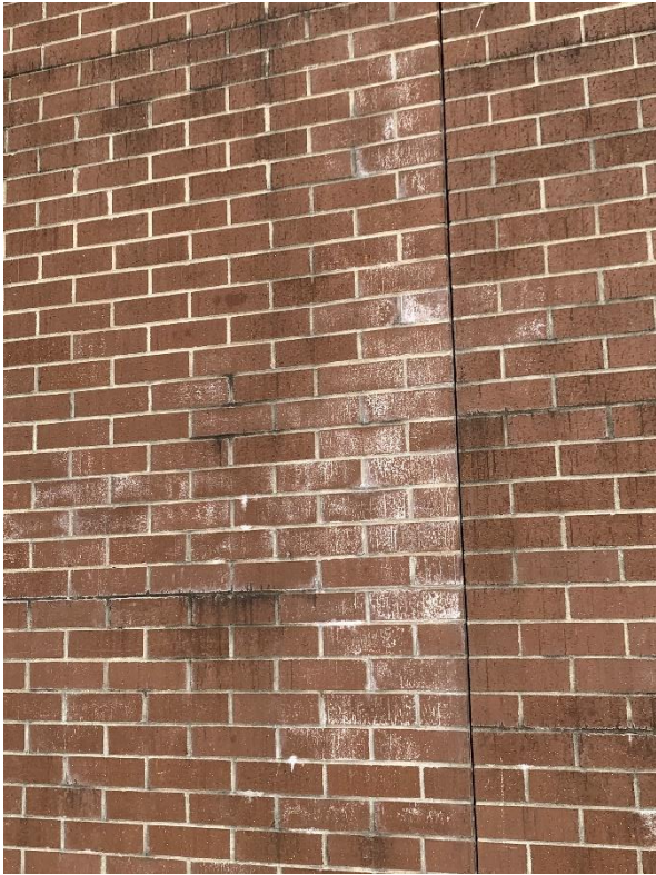
Efflorescence on brick veneer.
