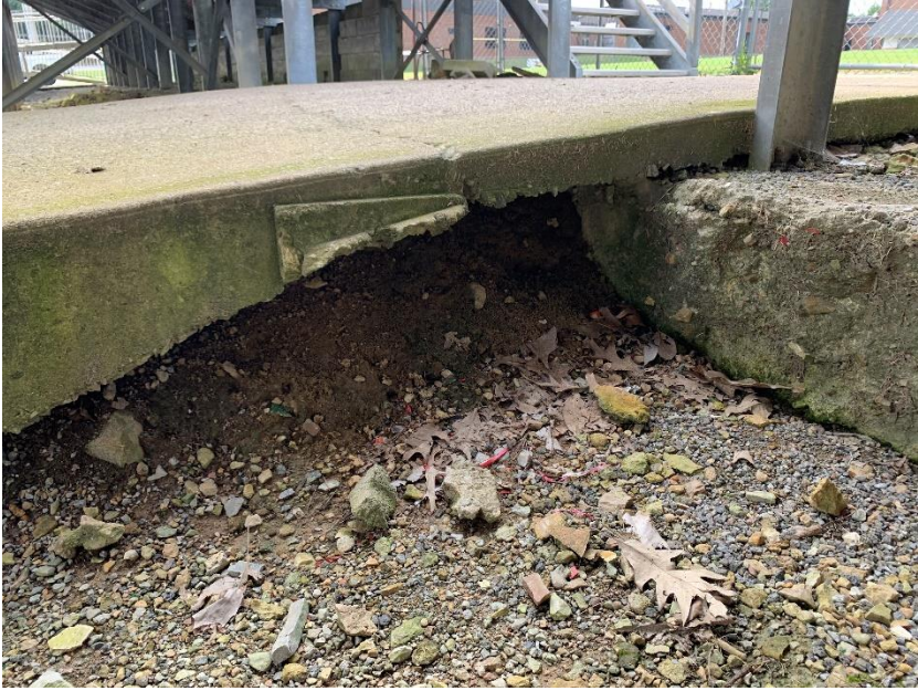
Undermining of concrete walkway at center entrance to Home side bleachers.
